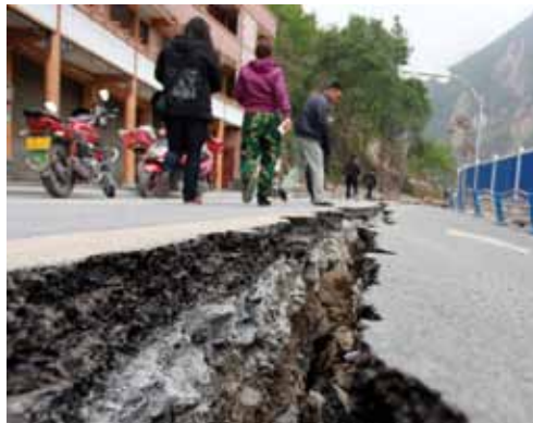
A total of 186 300 rural houses collapsed in the earthquakes in Sichuan
